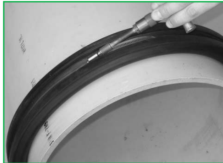
(Fig. 1) Tightening down one piece spliced WATER-STOP with torque wrench prior to grouting.
